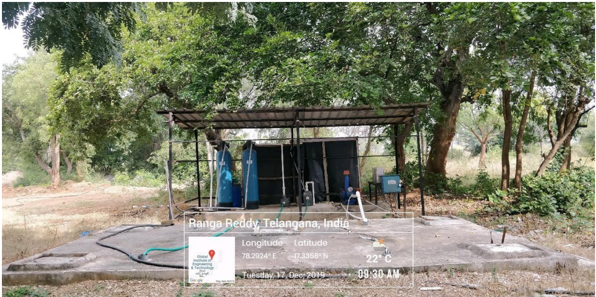
Sewage Treatment Plant in GIET Campus
